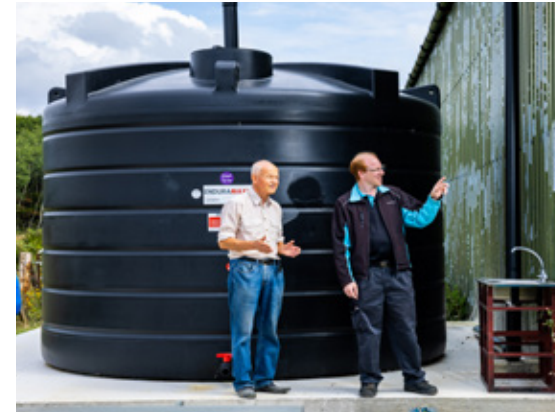
Rainwater harvesting system at a Sussex farm
