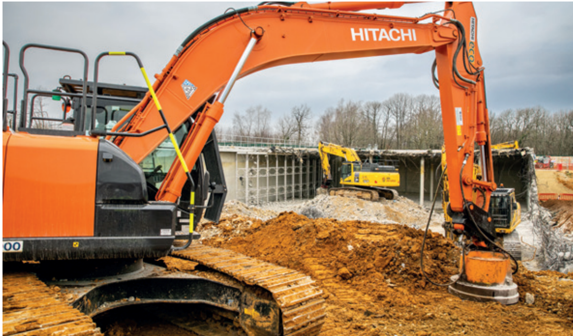
Butler Water Treatment Works, Kent
