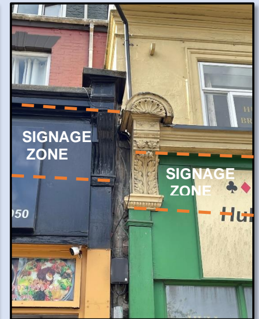
Figure 107 - 115-117 Spring Bank showing how the depth of the signage has increased beyond the original signage zone (Author, 2023)
