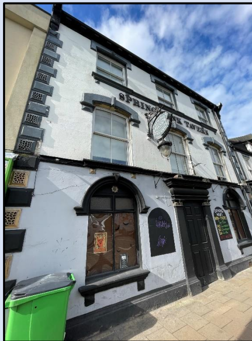
Figure 77 - Render utilised to the external walls of the Spring Bank Tavern (Author, 2023)
