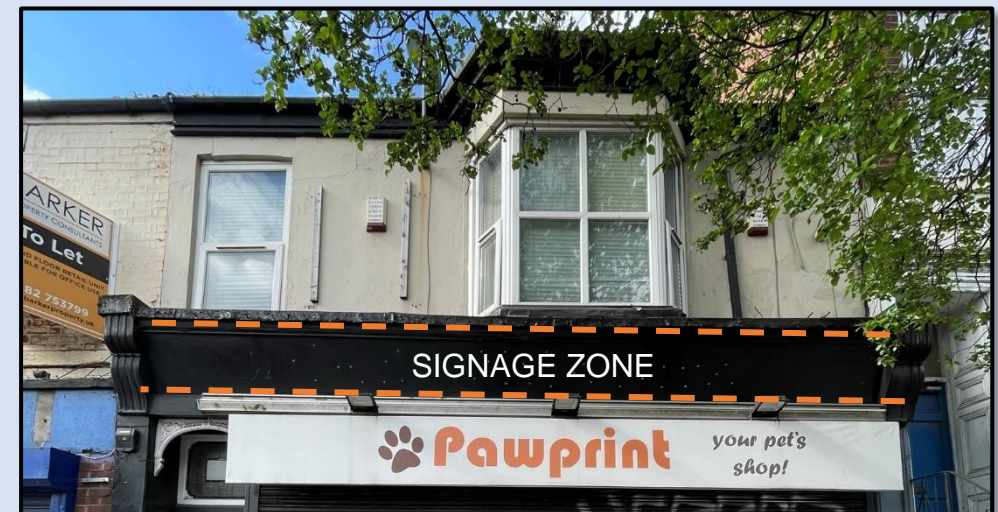
Figure 109 - 45 Spring Bank has retained its original fascia, cornice and corbels but the signage is positioned below the signage zone (Author, 2023)
